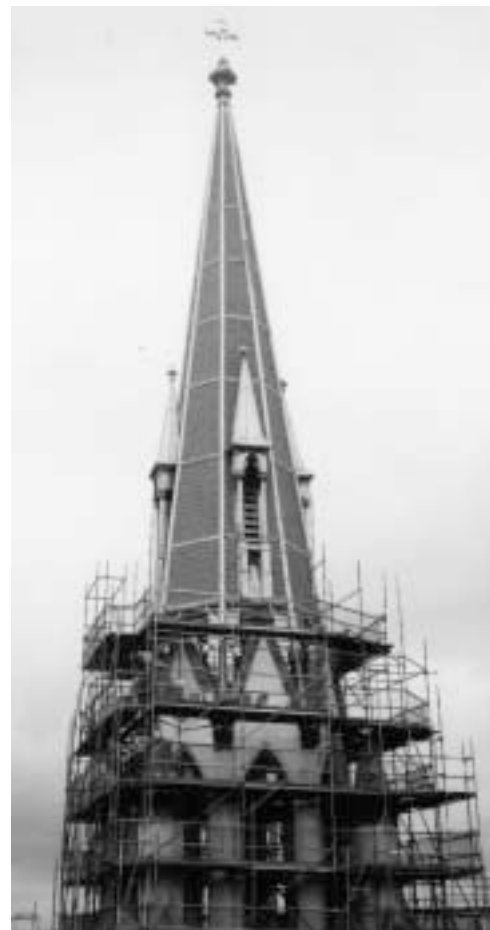
Spire of Saint John the Baptist Cathedral in Savannah, GA, restored by DPK&A Architects.
