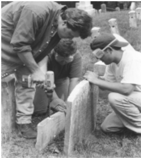
Building conservators Joan Berkowitz (center) and Ward Dennis (left) of Jablonski Berkowitz Conservation, Inc., carefully insert metal rods into vandalized gravestones in order to reset them. They later used a sand mixture colored to match the stone and remove signs of breakage. Sandy Ground Cemetery, Staten Island.
